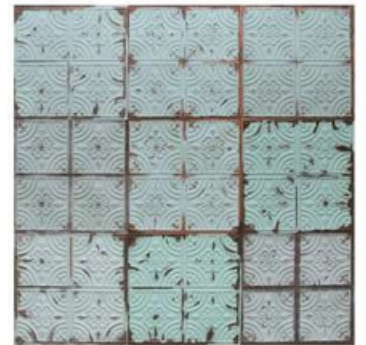
205 - Damaged Tin - 9 Tile Layout
